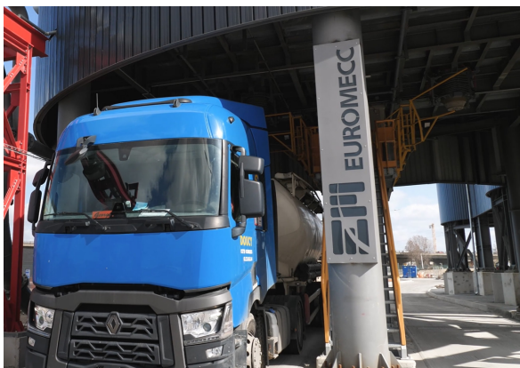
Every silo is designed to feed cement tankers with movable and retractable loading spouts.
