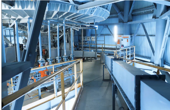
Under the discharge cone, it is possible to see all the pneumatic equipment.
